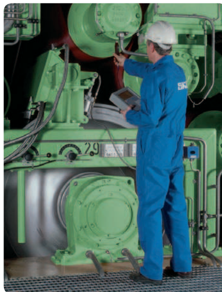
Checking vibration levels
